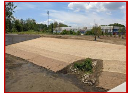
Erosion blankets and loose straw are used to protect seed while germinating. The erosion blanket nearest the water is made of coconut fiber which is more resistant within high water flow areas.
