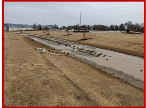
A rain basin is protected with erosion blankets while seeds are dormant underneath.
