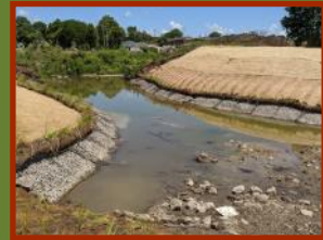
Erosion blanket and coir logs are installed to protect seed and native plugs within a high water flow area.
