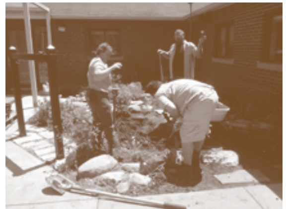
Volunteers install a rain garden at Fort Benjamin Harrison with help from the Fall Creek Watershed Project.
