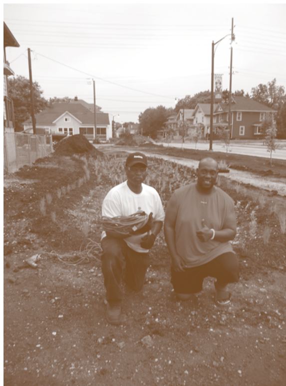
James Whitfield and Shawn Smith Sr. giving the thumbs up of approval for a rain garden installation and conservation practice well done! Finishing touches of mulch, pathway material and additional perimeter plantings are to be completed in phase II.
