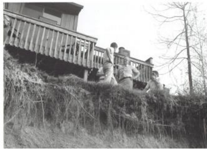
1982- District Conservationist Tom Pugh consults on severe streambank erosion problem
