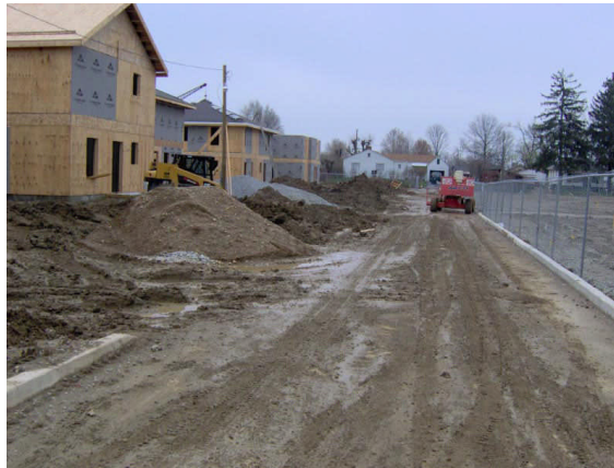
Soil in the street from a construction site
